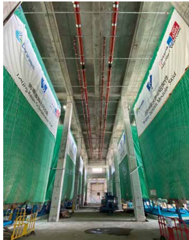
Reverse Osmosis Building—the heart of Tseung Kwan O Desalination Plant
